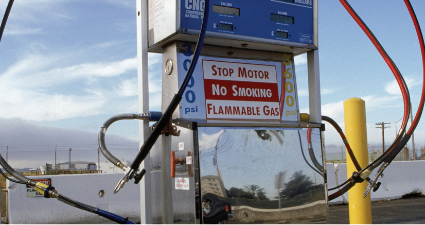
Compressed Natural Gas Dispensing
